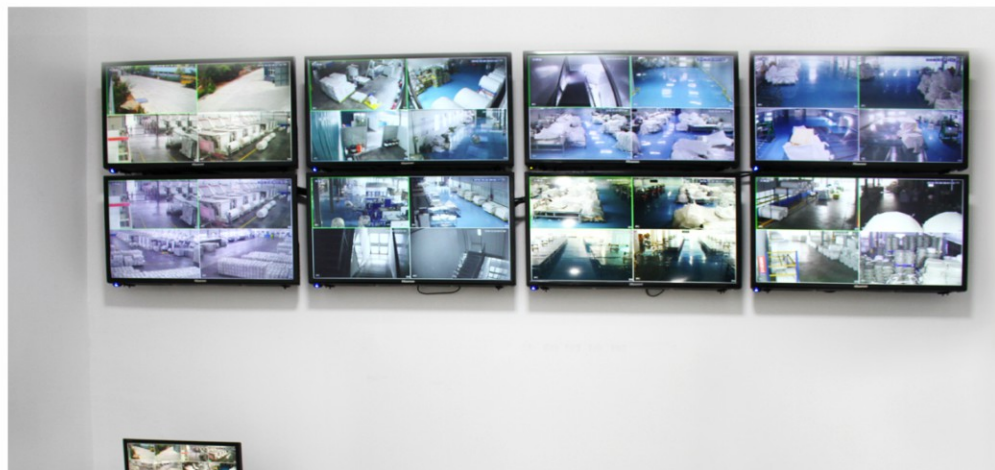
监控系统 Monitoring system
